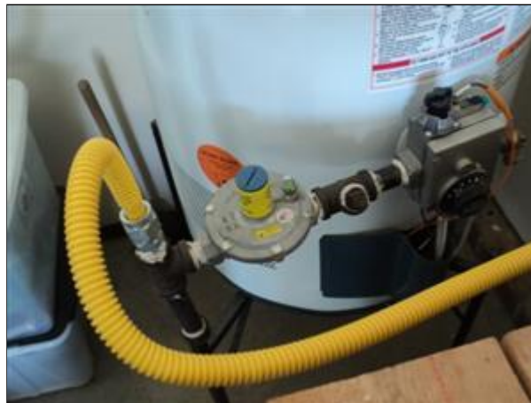
6.2 Picture 1 Hot water heater
