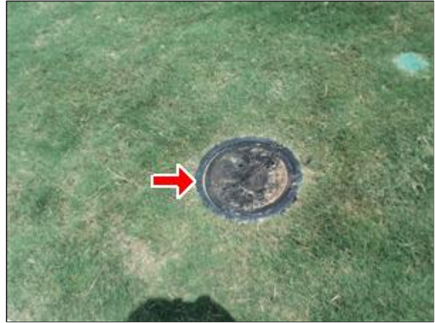
6.3 Picture 2 Water meter front yard
